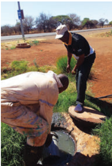
Community members used buckets to empty the overflowing manholes.
